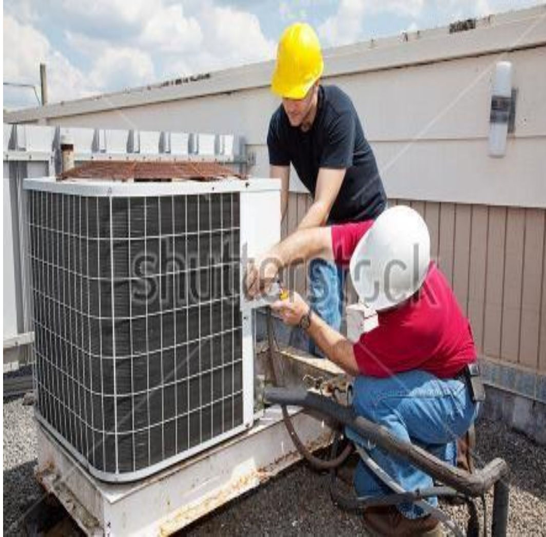
HVAC OUTDOORS UNITS MAINTENANCE
